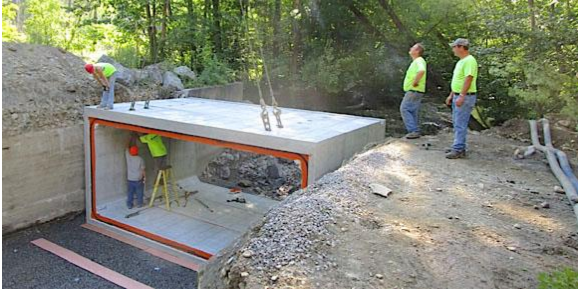
Tom Beach and Brian Sidle oversee the placement of a box culvert. (Photo provided)
